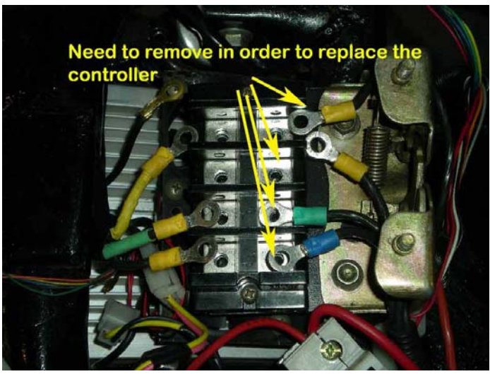
Picture shows controller wires.
